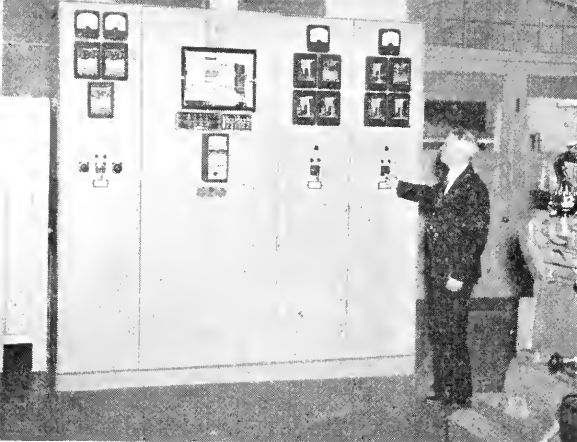
The newly-installed switchboard at the main pumping station
