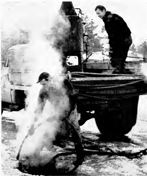
Opening frozen sewer at Chase and Drew Streets. David Feathers and Watson Burk on truck.
