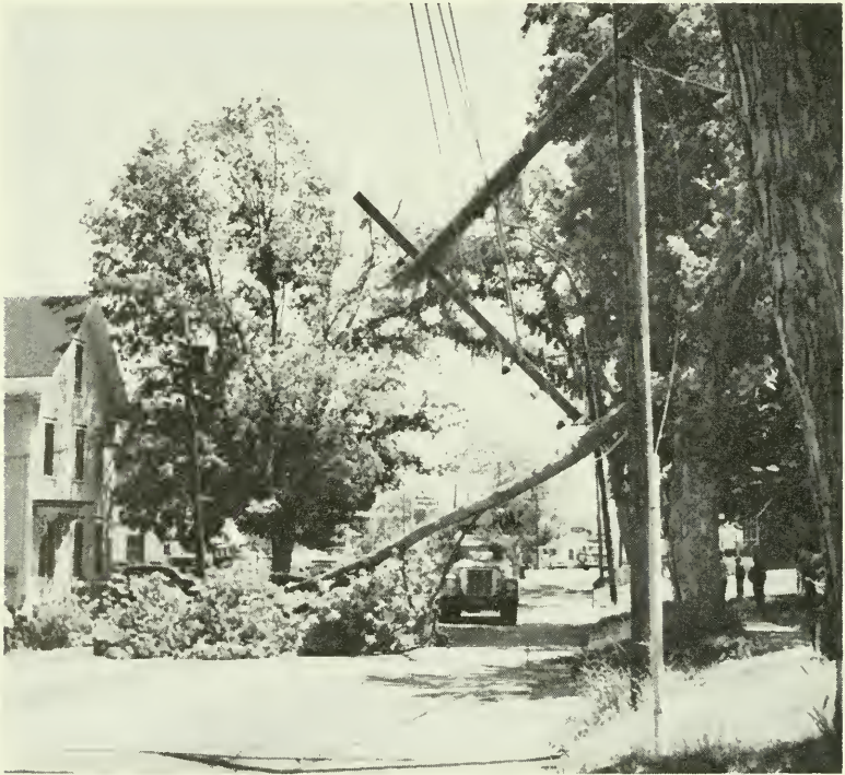
High winds caused this limb to fall bringing down cables and snapping off pole. Penacook CD Rescue Squad assisted Power Company employees at scene by roping off area, keeping pedestrians away, and directing traffic.
