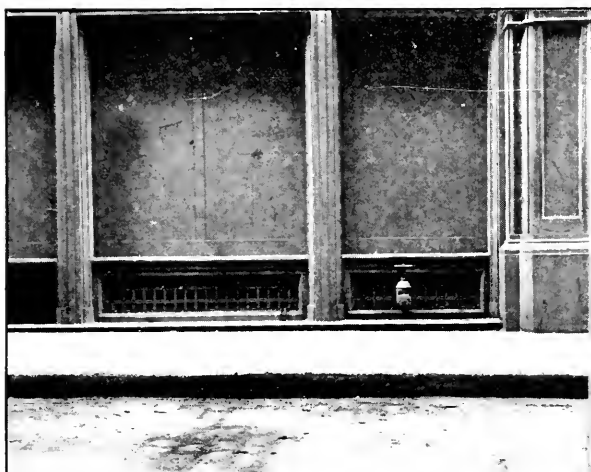
FIG. 1.— UNSCREENED BASEMENT VENTILATOR.
