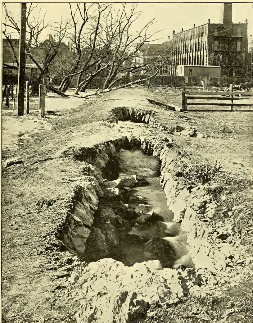
DORCHESTER-BROOK SEWER, — SHOWING NECESSITY OF BEING REBUILT.
