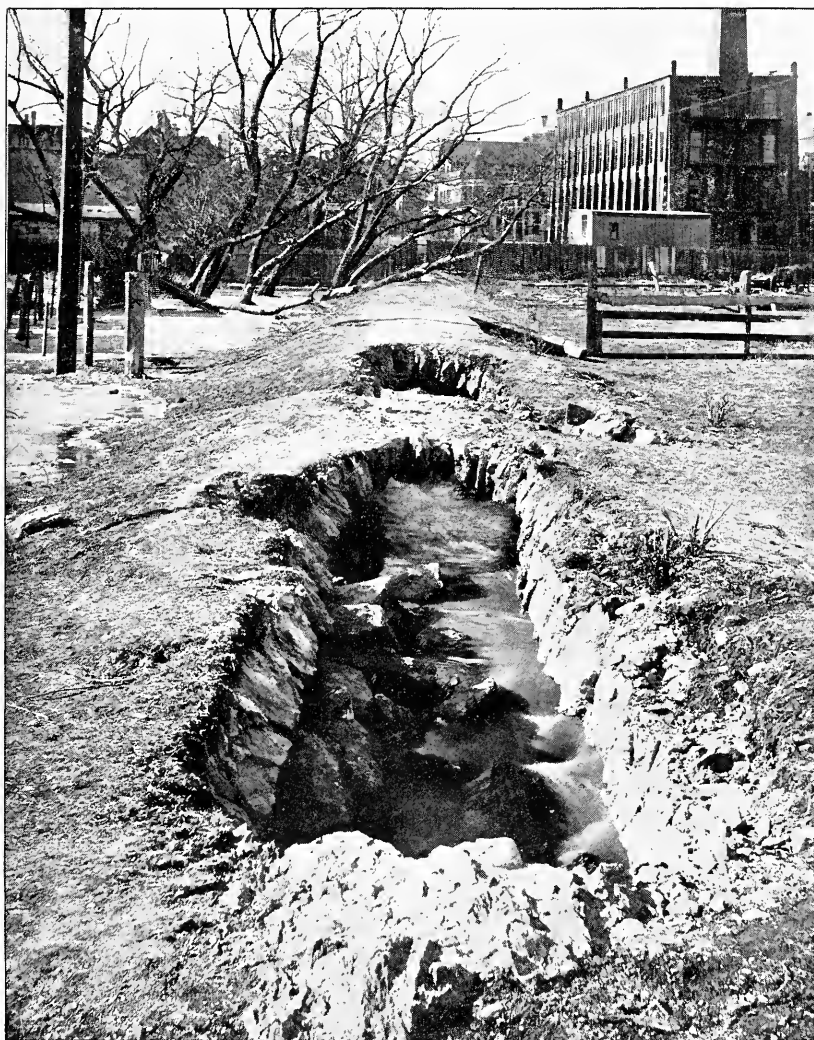
DORCHESTER-BROOK SEWER,—SHOWING NECESSITY OF BEING REBUILT.
