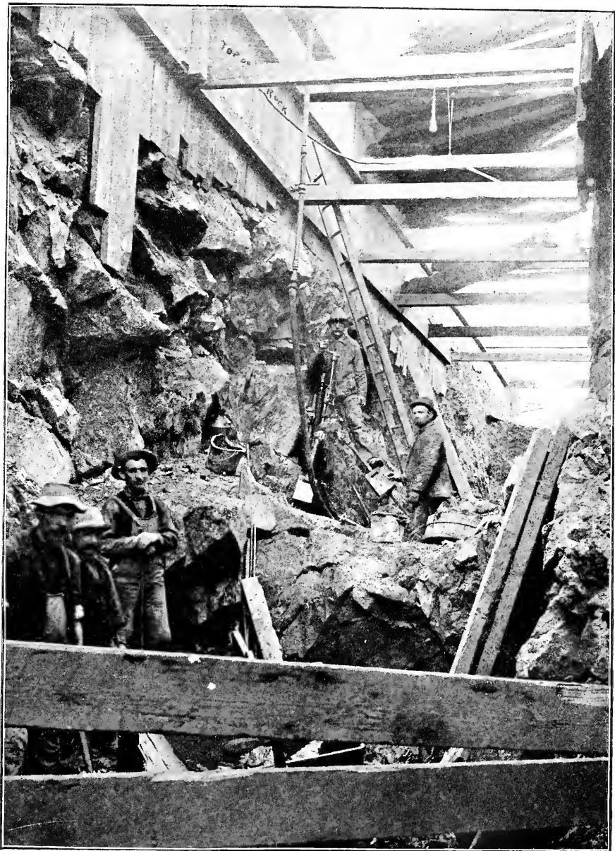
BLUE HILL AVENUE, DORCHESTER, SURFACE DRAINAGE. This surface drain will outlet into the Neponset river at Mattapan square.
