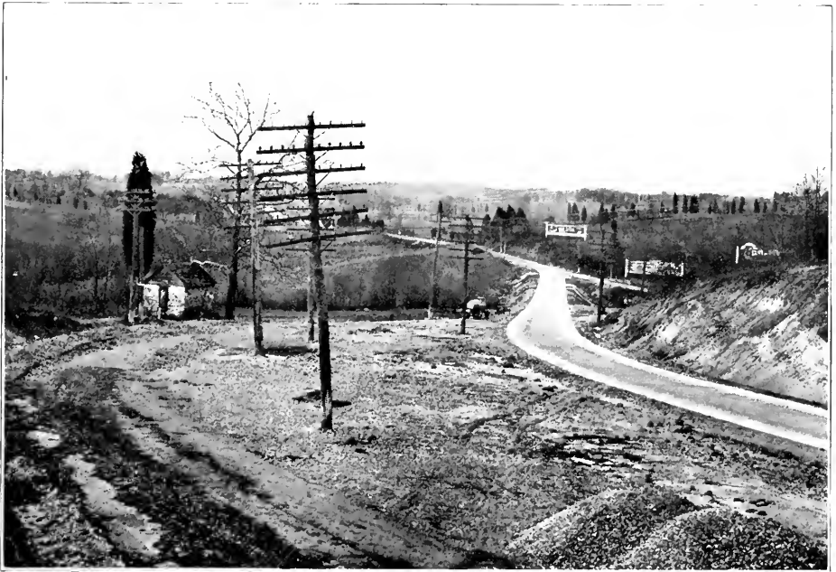
GENERAL VIEW OF THE ELIMINATION OF DEAD MAN'S CURVE ON THE BALTIMORE AND WASHINGTON BOULEVARD, LOOKING SOUTH.
