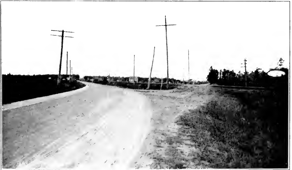
VIEW SHOWING ELIMINATION OF GRADE CROSSING ON WESTOVER-POCOMOKE ROAD, NEAR COSTEN, IN SOMERSET COUNTY.
