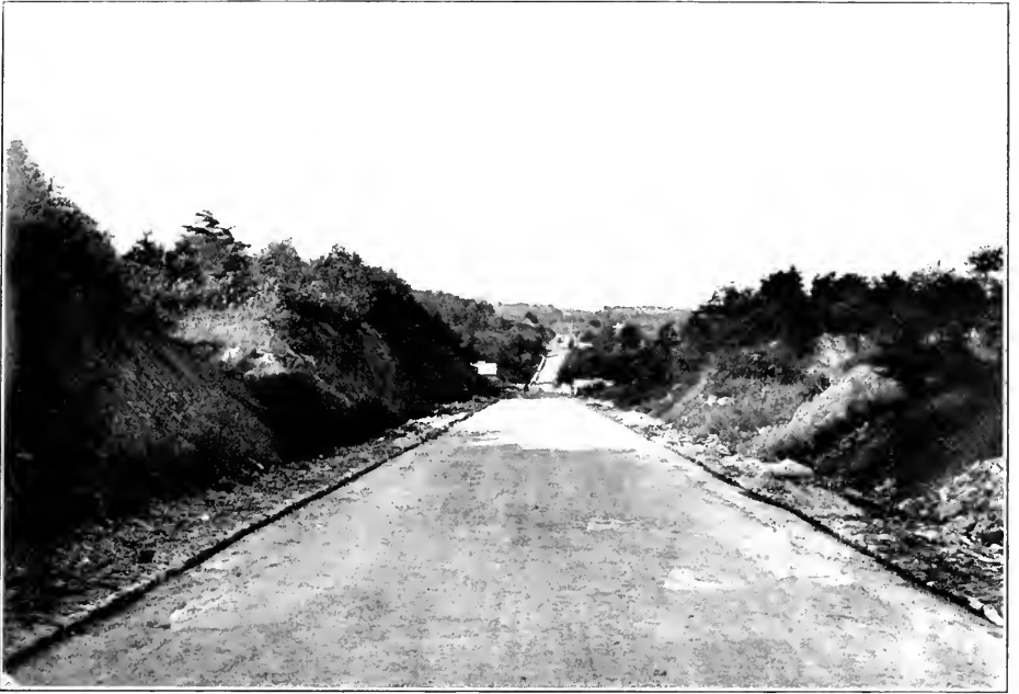
VIEW OF CONCRETE BASE, WITH COBBLE SHOULDER IN PLACE ON EACH SIDE, PRIOR TO SURFACING WITH SHEET ASPHALT. BALTIMORE AND WASHINGTON BOULEVARD, IN BALTIMORE COUNTY.
