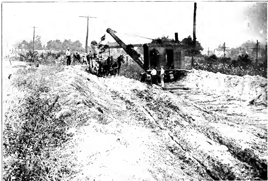
VIEW SHOWING STEAM SHOVEL AT WORK GRADING RELOCATION OF URBANA TURNPIKE, IN FREDERICK COUNTY.
