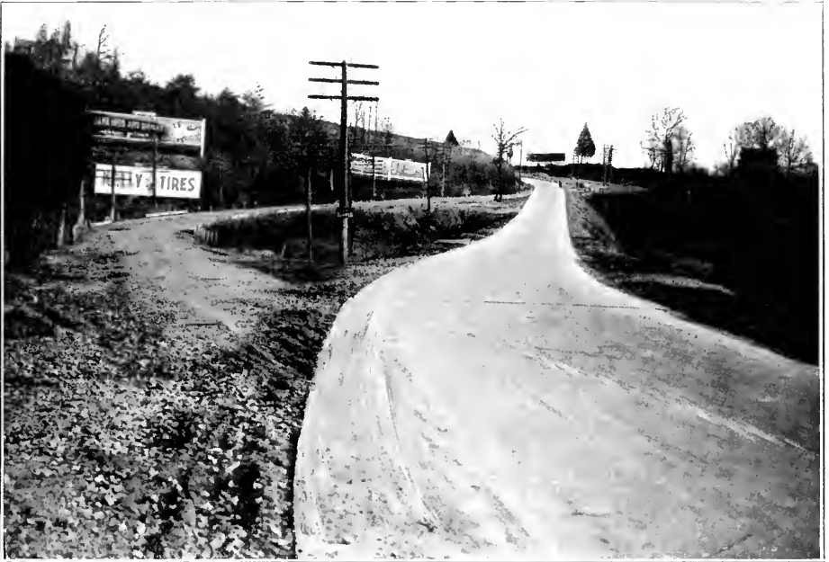
GENERAL VIEW OF THE ELIMINATION OF DEAD MAN'S CURVE ON THE BALTIMORE AND WASHINGTON BOULEVARD, IN HOWARD COUNTY, LOOKING NORTH.
