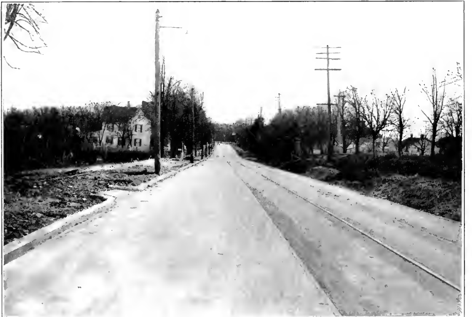
VIEW OF STREET IN REISTERSTOWN, SHOWING FINISHED CONCRETE ROADWAY, WITH COMBINATION CURB AND GUTTER ON LEFT AND STEAM SHOVEL GRADING ON RIGHT.
