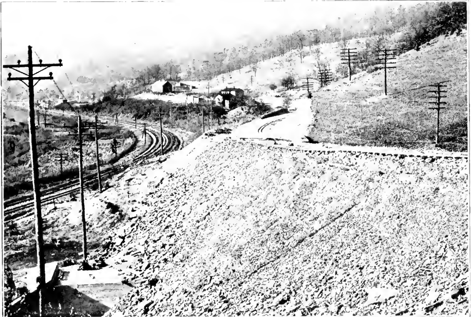
VIEW SHOWING FORTY-FOOT FILL, CONCRETE CULVERT AND BEGINNING OF CONCRETE ROADWAY ON McMULLEN HIGHWAY, IN ALLEGANY COUNTY, LOOKING WEST FROM STATION No. 46.
