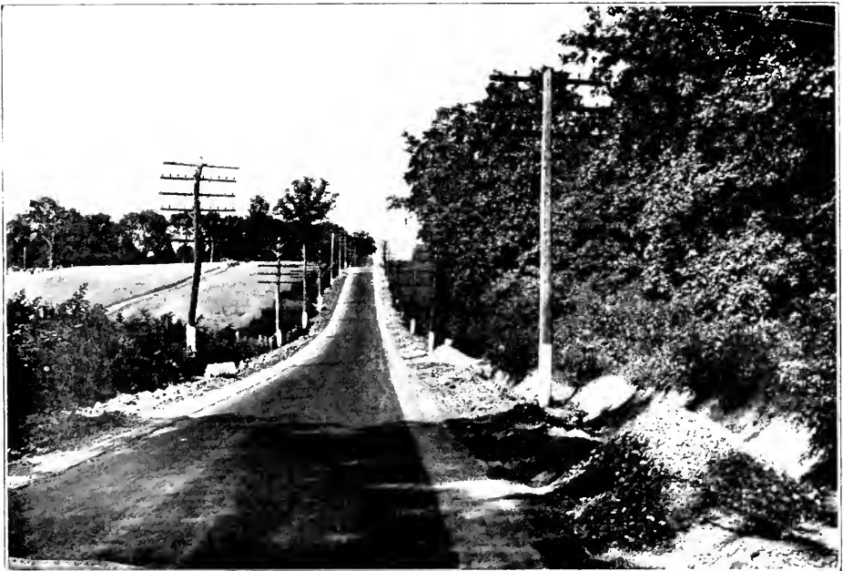
GENERAL VIEW SHOWING CONCRETE SHOULDERS ON BELAIR ROAD, IN HARFORD COUNTY. MACADAM ON LEFT NOT YET FILLED IN AGAINST SHOULDER.
