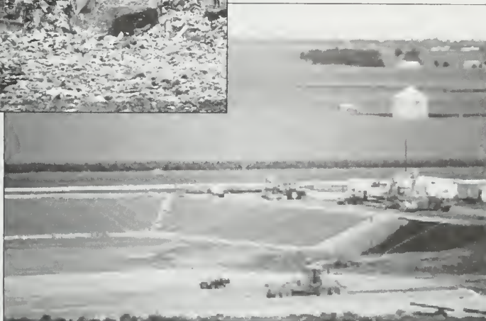
Waste landfill near Sreator. Geologic information is essential for identifying underlying strata that will contain pollutants and protect the groundwater.
