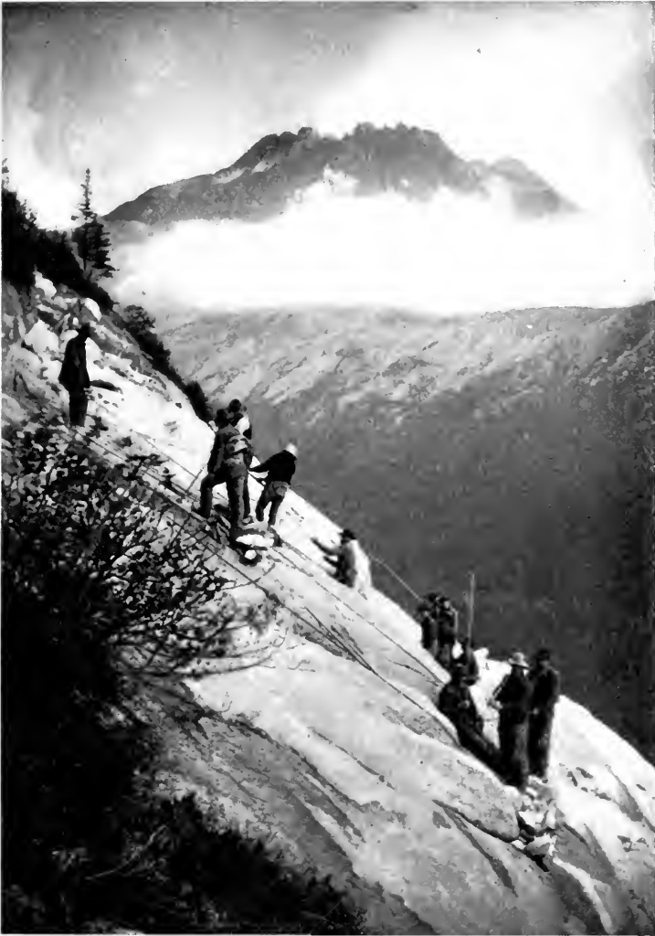
CUTTING GRADE FOR THE PACIFIC AND ARCTIC RAILWAY—TUNNEL MOUNTAIN, WHITE PASS ROUTE.
