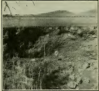
FIG. 2(b). Headcut of Willow Creek gully, tributary of Milk River near Glasgow, Montana. Height 25 feet. Hay meadow directly above.
