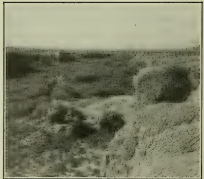
FIG. 5(c). Gradual filling in unnamed gully north of Shiprock, New Mexico. Looking downstream. Depth of fill at lower end more than 6 feet.
