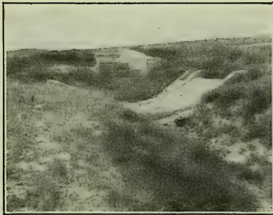
FIG. 6(c). Spillway and drop structure leading from spreader dike constructed by C.C.C. Steamboat demonstration area, Navajo Indian Reservation near Ganado, Arizona. Structures have prevented deepening of the channel but will soon fail unless repaired.
