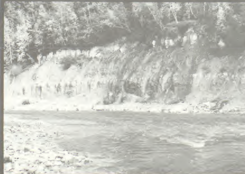
Unstable bank at km 13.9.
