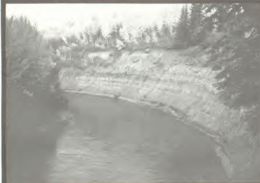
Long section of eroded bank at km 22.
