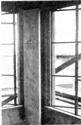
Steel sash with plastered reveals and tile studs. Corner cupboard in wall-hollow with pivoted Fabricrete door.
