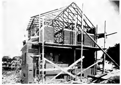
Steel frame in place and part of the outer brick work in position
