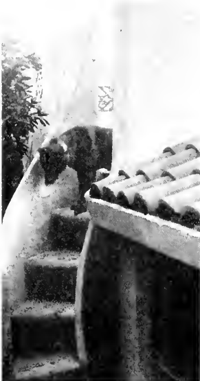
Spiral stair to roof terrace, treads, risers and rails made of stucco. The terrace parapet also of stucco. The terrace parapet also of stucco, is about 1 1/4" thick, 4" high and 8" long, reinforced with netting and 3/8" rods. Tests have proven that it has ample strength.
