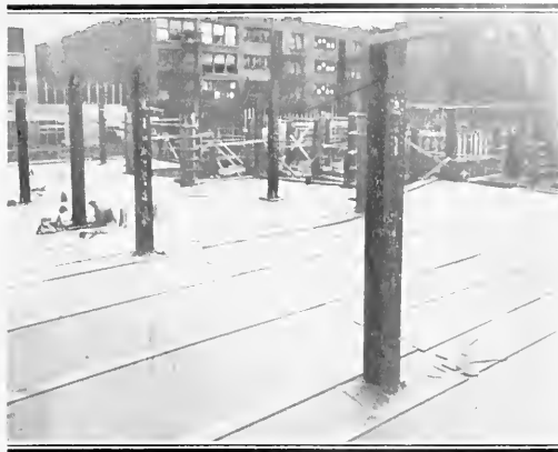
10,000 sq. ft. of Sisalkraft were used for curing and protecting the concrete floors of this department store in Vancouver
