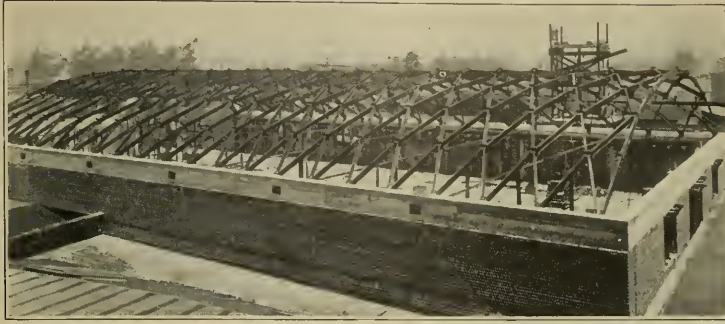
STEEL LAMELLA ROOF, COCO COLA PLANT, LOS ANGELES. THIS ROOF HAS A 70-FOOT SPAN
