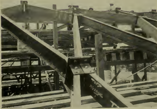
BRACKETS RIVETED TO ENDS OF STEEL CHANNEL LAMELLAS AND BOLTED TOGETHER THROUGH STEEL PLATES
