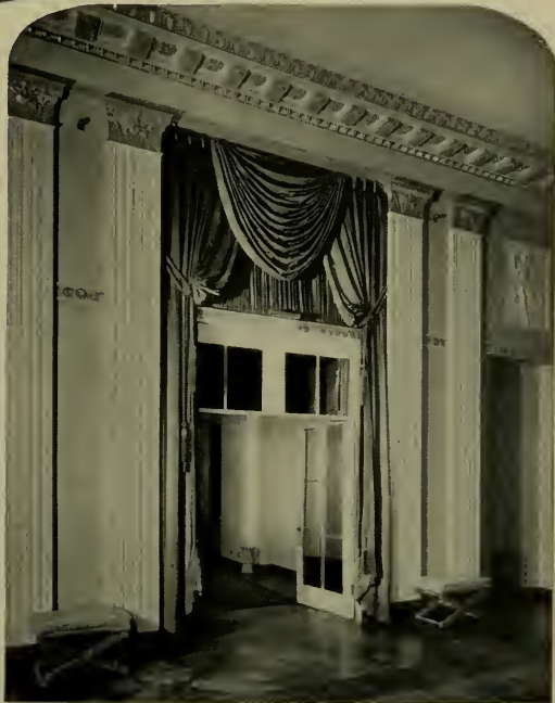
The curtain above this doorway in one of the public rooms of the Waldorf-Astoria conceals a loudspeaker
