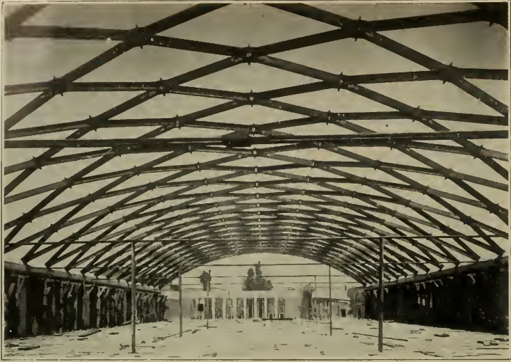
INTERIOR VIEW OF ROOF CONSTRUCTION, SHOWING STEEL TRUSSES BEFORE ENCASED IN CONCRETE
