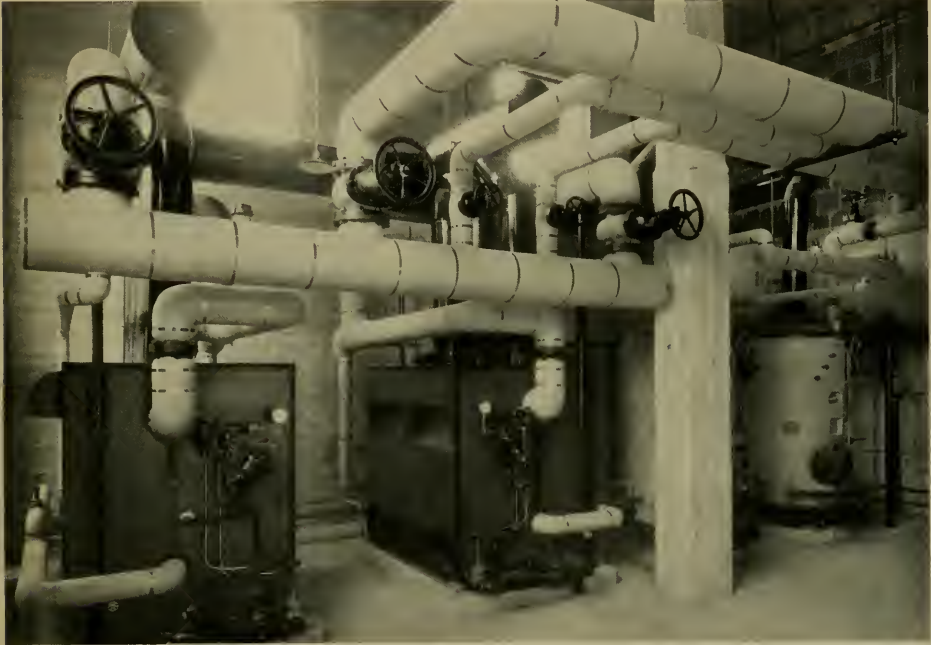
INTERIOR OF BOILER PLANT, ST. BERNARDINE HOSPITAL I. E. Loveless, Architect and Engineer
