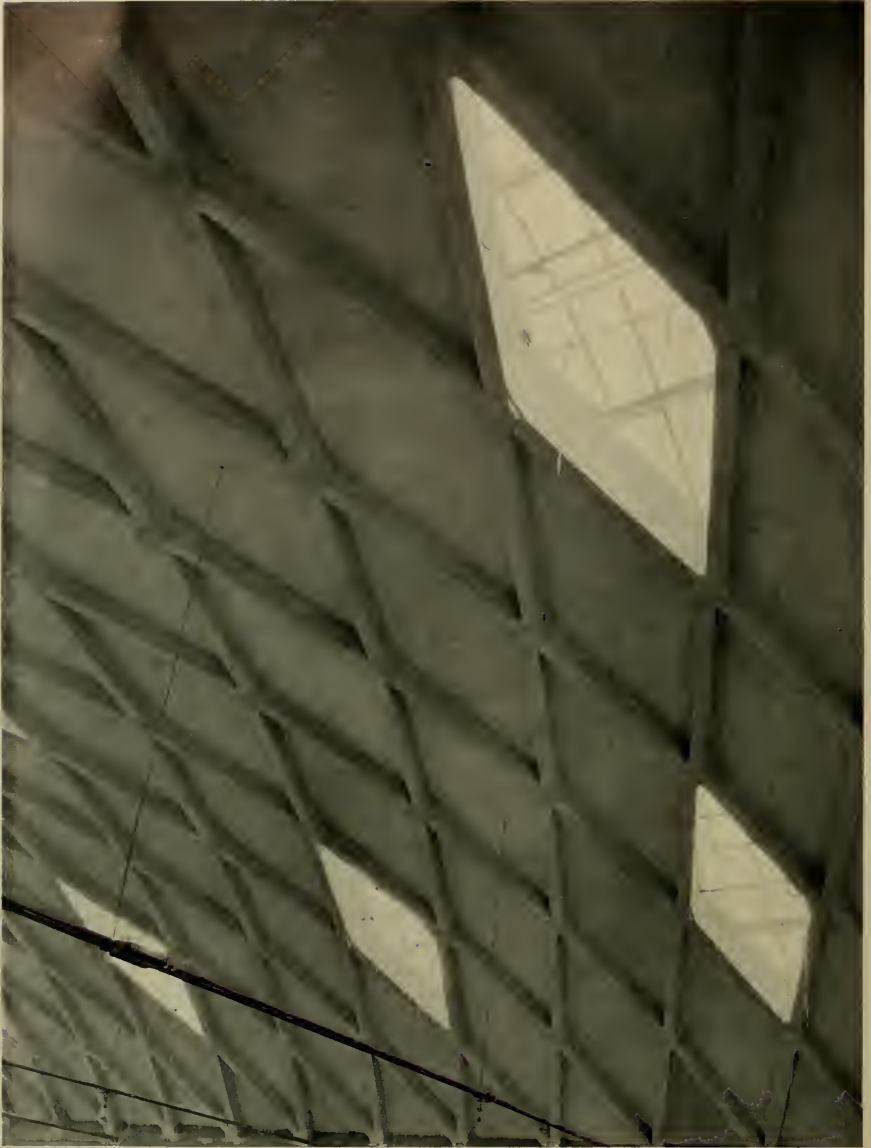
CLOSE UP OF ROOF CONSTRUCTION, COCO COLA WAREHOUSE STEEL MEMBERS FIREPROOFED WITH TWO INCHES OF CONCRETE
