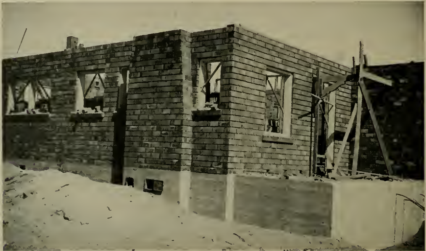
BOULDER CITY, NEVADA Typical residence showing stripped joints in brickwork.
