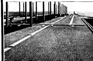
STEELEX Floor Lath is unrolled over the joists. The illustration above shows STEELTEX Floor Lath in an unbroken stretch of 212'.
