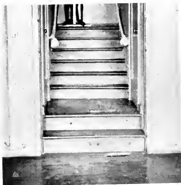
Fig. 2—The floor and stairs shown in Fig. 1 were found to have been gutted by these pests
