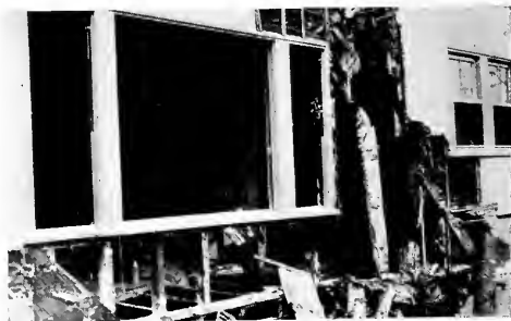
Fig. 4—The collapse of the wall and entrance of this home showed it to have been gutted by termites
