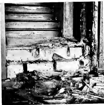
Fig. 1—There was no visible evidence of the presence of termites until the floor in the foreground was punctured by a high heel.
