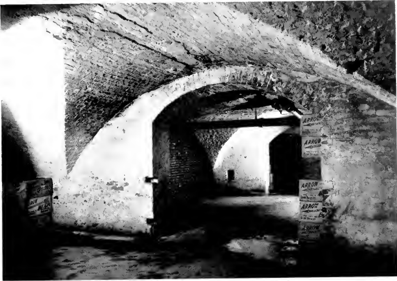
ALTHOUGH NEARLY 200 YEARS OLD, THESE VAULTS IN GLOBE BREWERY, BALTIMORE, ARE STILL IN SPLENDID CONDITION
