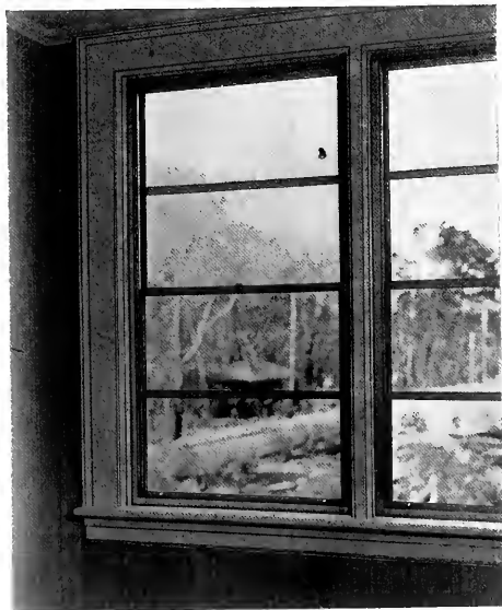
Installation completed and trim applied. Note narrow mullion and unobtrusive hardware. Sash may be raised or lowered with little finger.
