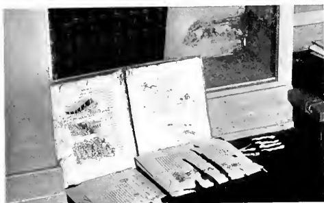
Fig. 3—The hazard in building an unprotected structure near a termite colony is very real. Within four months after his home was completed this damage was done.
