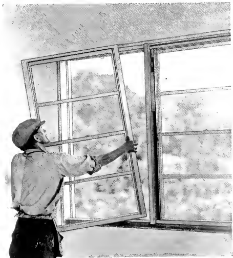
Carpenter attaches metal frame to simple wood sub-frame using ordinary wood-screws. Removable strip makes weights easily accessible.
