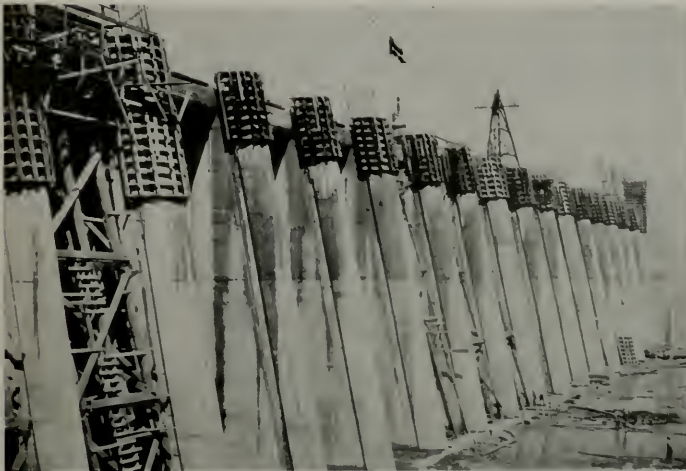
A recent photograph of the power-house dam, across the river channel on the Oregon side. The view is of the upstream face; during construction the water of this channel has been diverted. The power-house at this point will generate 115,000 horsepower, or 86,000 kilowatts; later this output may be doubled.
