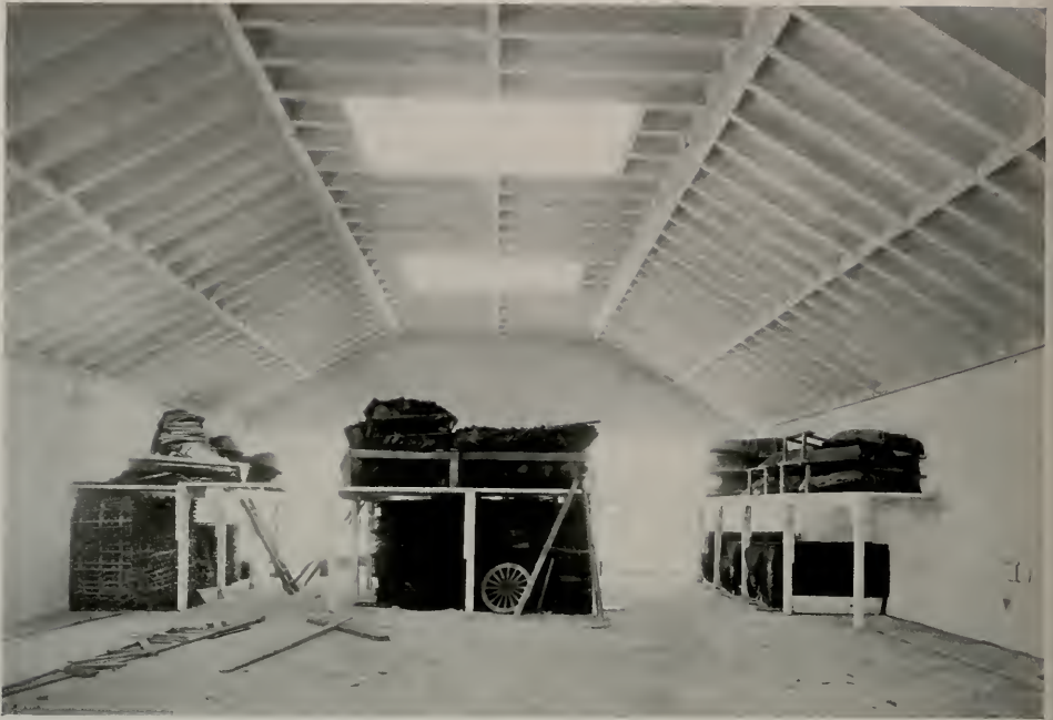
INTERIOR REINFORCED CONCRETE BUILDING FOR STEEL FORM CONTRACTING COMPANY, SAN FRANCISCO, SHOWING NEW TYPE OF ROOF CONSTRUCTION. L. H. Nishkian, C.E.
