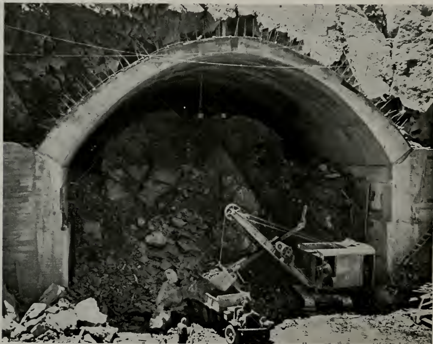
DOWN TO THE CORE. With the tunnel completely concreted and steel lined by novel construction methods, a steam shovel begins removal of thousands of cubic yards of rock from 58 by 76-foot bore. Article on Page 58.
