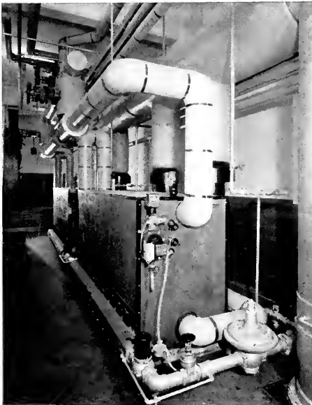
GAS FIRED BOILER PLANT IN SUNKIST BUILDING, LOS ANGELES
