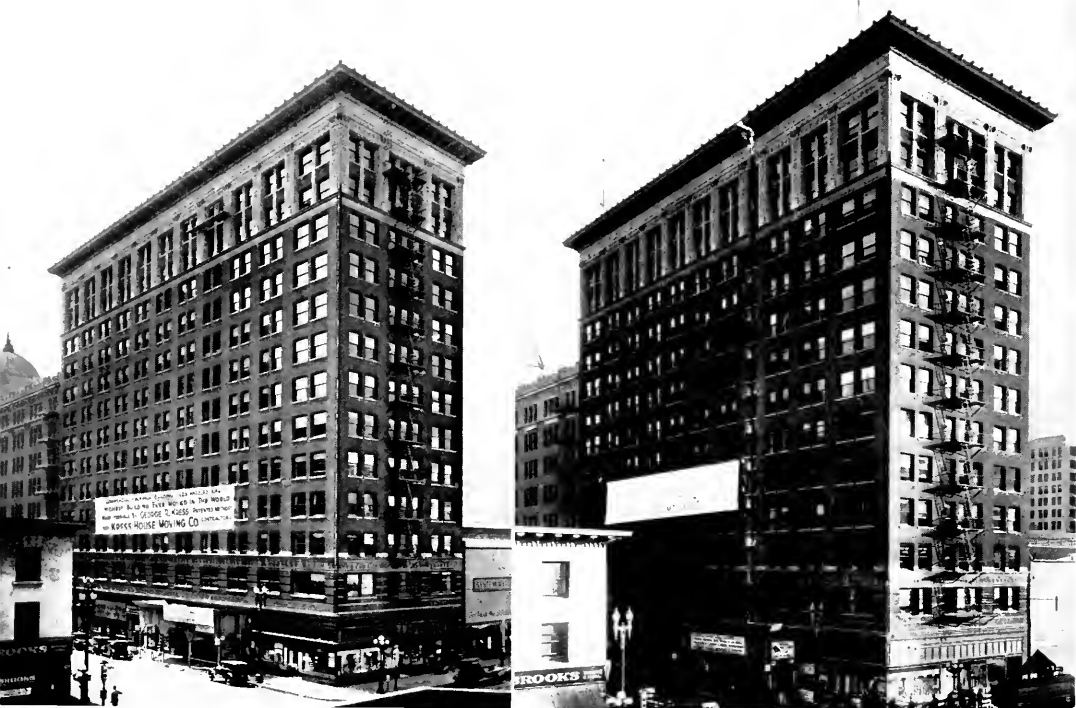
Commercial Exchange Building, Los Angeles. Picture on left shows building before cut in two; Photo on right shows appearance of building after rejoining the two sections.
