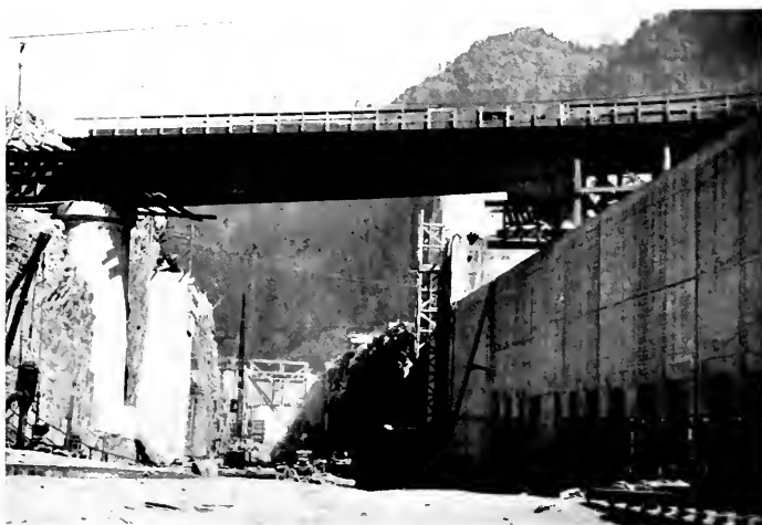
One view of the navigation locks being built between Bradford Island and the Oregon shore of the river. Above is seen the present Union Pacific Railroad right-of-way. The tracks of this line will be relocated, moved higher up the canon slope so big ships may pass where trains now run.
