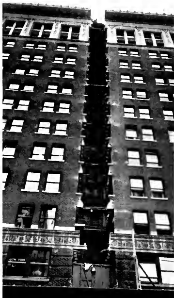
Commercial Exchange Building, Los Angeles, as it appeared after an 8½ ft. slice had been cut out of the structure. (Courtesy Southwest Builder and Contractor)
