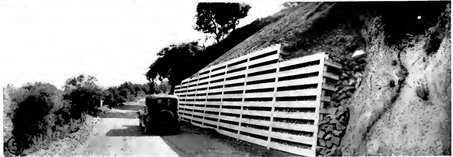
METAL CRIBBING PROVIDES EXCELLENT RETAINING WALL FOR COUNTY HIGHWAY NEAR MORAGA, CALIFORNIA 1—Preliminary excavation for the wall. 2—Placing the first course of cribbing units on correct line and batter. 3—Assembling or erecting the cribbing courses. 4—Cribwall complete, ready for the remainder of the backfill. 5—Completed job. The roadway above at the right can be visualized.
