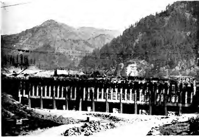
The power-house dam as seen from the downstream side. Over the roads in the foreground constantly roll Standard Oil trucks with fuel and lubricants used by the contractors. When the project is completed, these roads will be buried beneath water flowing through the power-house above the dam.
