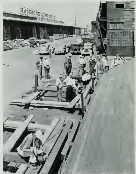
APPLYING LATERAL LOAD ON WEST SILL ONLY BY MEANS OF HYDRAULIC JACKS. DISTRIBUTING BEAM SYSTEM FOR EVEN APPLICATION OF LOAD TO SILL IS SEEN IN FOREGROUND.
