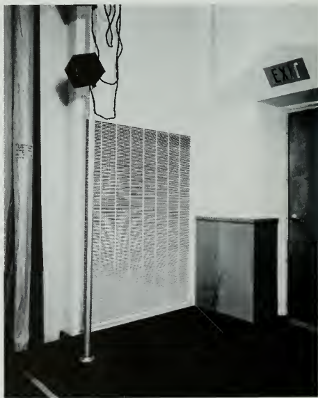
CORNER OF THE STAGE OF STUDIO D, N. B. C.'S NEW HOLLYWOOD RADIO CITY. THE GRILLING HIDES A HUGE AIR DUCT
