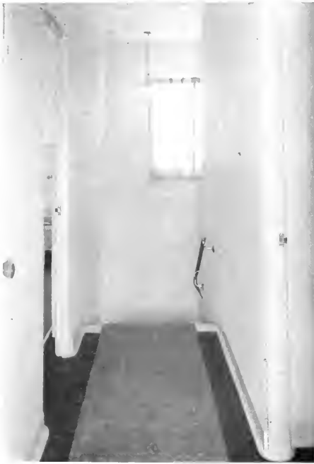
INTERIOR VIEW OF ALAMEDA CONCRETE HOUSE, showing trim and base moulds in cast concrete.
