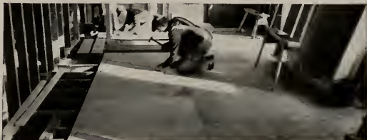
SUB-FLOORING In this Stamford, Conn., home designed by Provost and Edwards, Plyscord provided a smooth base for finish flooring and linoleum—insulates and protects against drafts from below—gives a horizontal diaphragm to resist earthquakes and high winds. Recommended thicknesses are 1/2" and 5/8".
