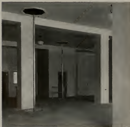
"Monterey Buff" was selected as the color for this installation which assures resistance to fire, acid stains, moistures, and other hard usage and at the same time affords a surface easy to clean and one that need never be painted or otherwise reconditioned.
