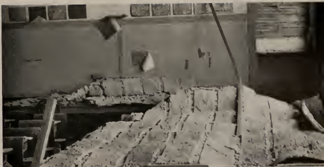
CEILING DROPPED TO FLOOR IN ONE OLD SCHOOL BUILDING
