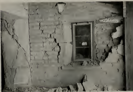
TOP AND LOWER PICTURES SHOW CRUMBLED ADOBE WALLS OF BRAWLEY CITY HALL. MIDDLE PHOTO SHOWS STEEL REINFORCING BARS PULLED OUT OF GIRDER. NOTE HOW TWO BARS IN GIRDER WERE DISCONTINUED AT SECTION OF MAXIMUM MOMENT.
