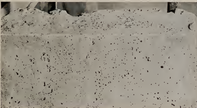
Surface voids disclosed by stoning the surface of a laboratory specimen cast under a sloping wood form. These voids are often hidden by a thin film of cement and fine sand; do not show up when forms are stripped in ordinary field operations.
