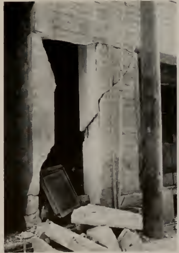
TOP PICTURE SHOWS SHATTERED ADOBE WALLS OF BRAWLEY FIRE HOUSE AFTER RECENT IMPERIAL VALLEY TREMOR. LOWER PHOTO SHOWS FAILURE OF POORLY DESIGNED CONCRETE WALLS.
