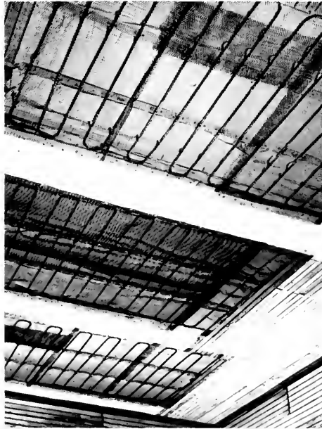
GAS-FIRED PANEL HEATING EQUIPMENT INSTALLED IN CEILING
