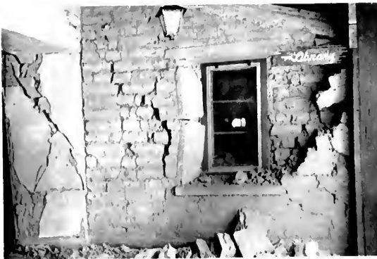
TOP AND LOWER PICTURES SHOW CRUMBLING ADOBE WALLS OF BRAWLEY CITY HALL. MIDDLE PHOTO SHOWS STEEL REINFORCING BARS PULLED OUT OF GIRDER. NOTE HOW TWO BARS IN GIRDER WERE DISCONTINUED AT SECTION OF MAXIMUM MOMENT.
