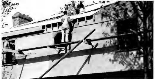
The Plyscord-sheathed walls of this residence in Seattle, Wash., are 40% more rigid than if diagonal board sheathing had been used. The big panels also save up to 80% on sawing, fitting and joining... 50% on nailing. Teanys Francis Bellomy was the architect on this residence.
