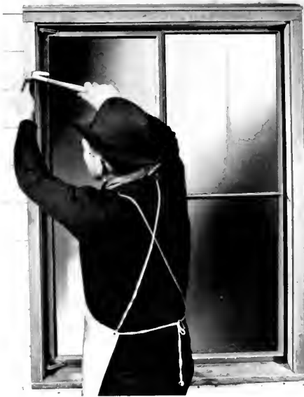
USING ONLY HAMMER AND NAILS, ANY CARPENTER CAN INSTALL THIS WINDOW IN LESS THAN FIVE MINUTES
