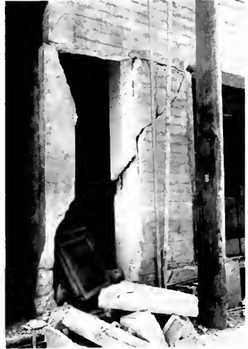
TOP PICTURE SHOWS SHATTERED ADOBE WALLS OF BRAWLEY FIRE HOUSE AFTER RECENT IMPERIAL VALLEY TREMOR. LOWER PHOTO SHOWS FAILURE OF POORLY DESIGNED CONCRETE WALLS.
