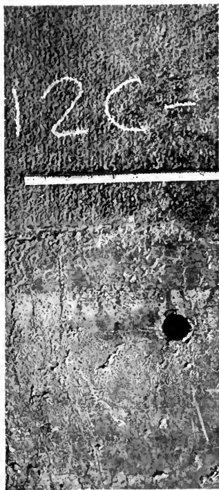
Field demonstration showing surface texture of concrete placed at Grand Coulee Dam test against absorptive lined forms at the top, as compared with concrete placed against wood forms, below.
