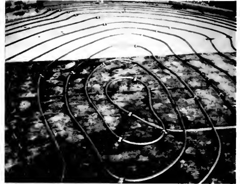
GAS-FIRED PANEL HEATING EQUIPMENT INSTALLED IN FLOOR
