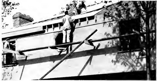
WALL SHEATHING The Plyscord-sheathed walls of this residence in Seattle, Wash., are 40% more rigid than if diagonal board sheathing had been used. The big panels also save up to 50% on sawing, fitting and joining... 50% on nailing. Tenney Francis Bellamy was the architect on this residence.
