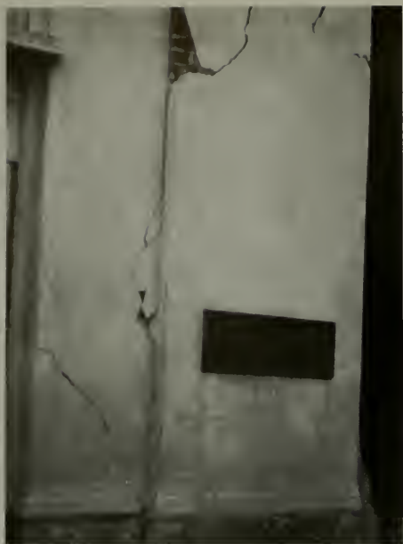
Looking northwest at Benjamin Franklin Life Building, Santa Barbara, California. Close-up of north side of entrance.
