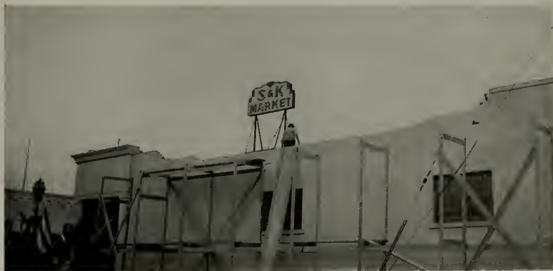
Looking west at S & K Market, State and Ortega Sts., Santa Barbara, California. Top of brick wall on southeast side of building fell.
