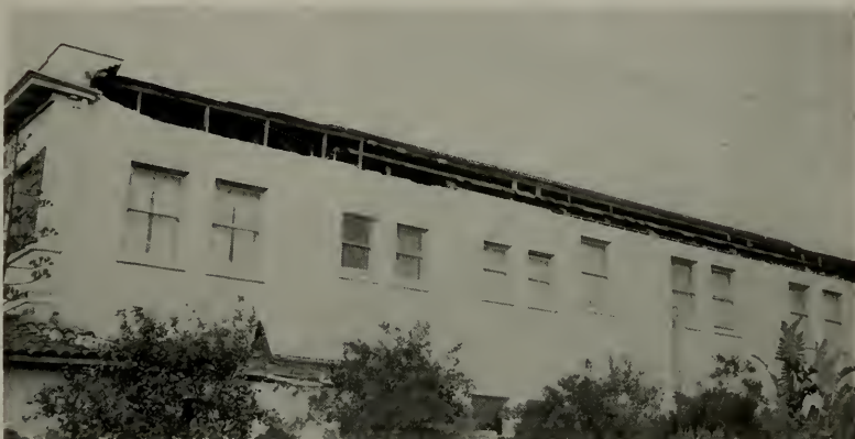
Looking south at Masonic Temple, Carpinteria. Top of northeast brick wall fell.
