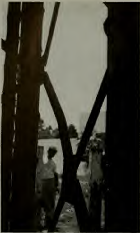
Water Tank, S.P. R.R., Santa Barbara, California. Showing bent diagonal in lower panel of steel tower. About a dozen diagonals were similarly bent.
