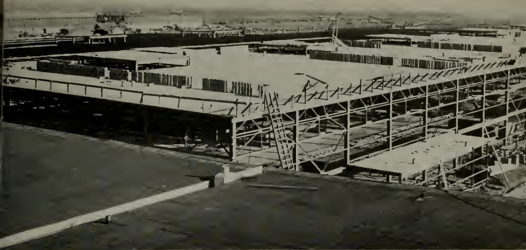
Progress picture of main assembly building (one of eleven) for the Douglas Aircraft Company, Inc., at North Long Beach, California.
