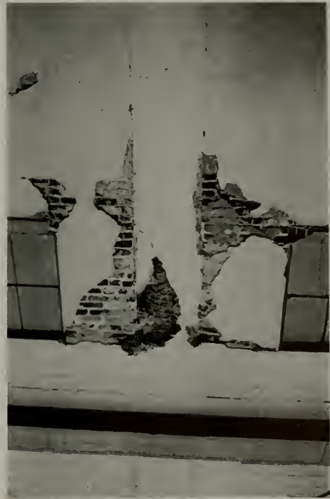
Looking northeast at Bekins Van & Storage Warehouse, Santa Barbara, California. Showing broken brickwork and possible cracked column.
