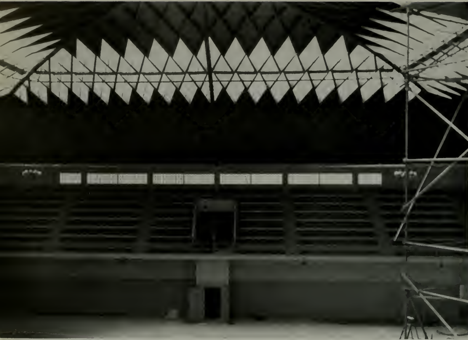
Interior of Union High School Gymnasium, Phoenix, Arizona, showing Lamella type of roof construction.
