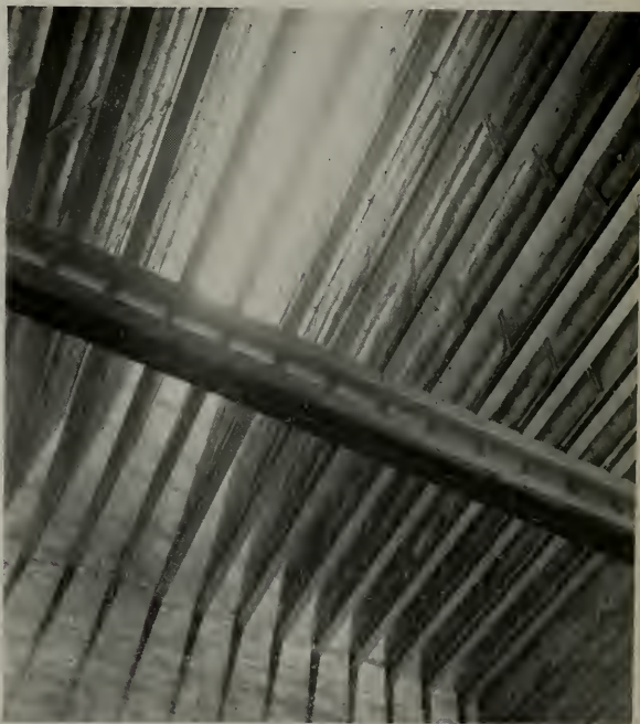
Interior view of inlet stack, looking up through the stack from a test cell floor, showing how Fiberglas bats are installed between metal sheets, and spacing of baffle plates.
