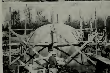
Construction methods: Pictured from top down—(1) Laying out the balloon form; (2) Method of anchoring; (3) Inflating canvas with compressed air; (4) Mounting window frames and dusting balloon so cement won't stick to it.
