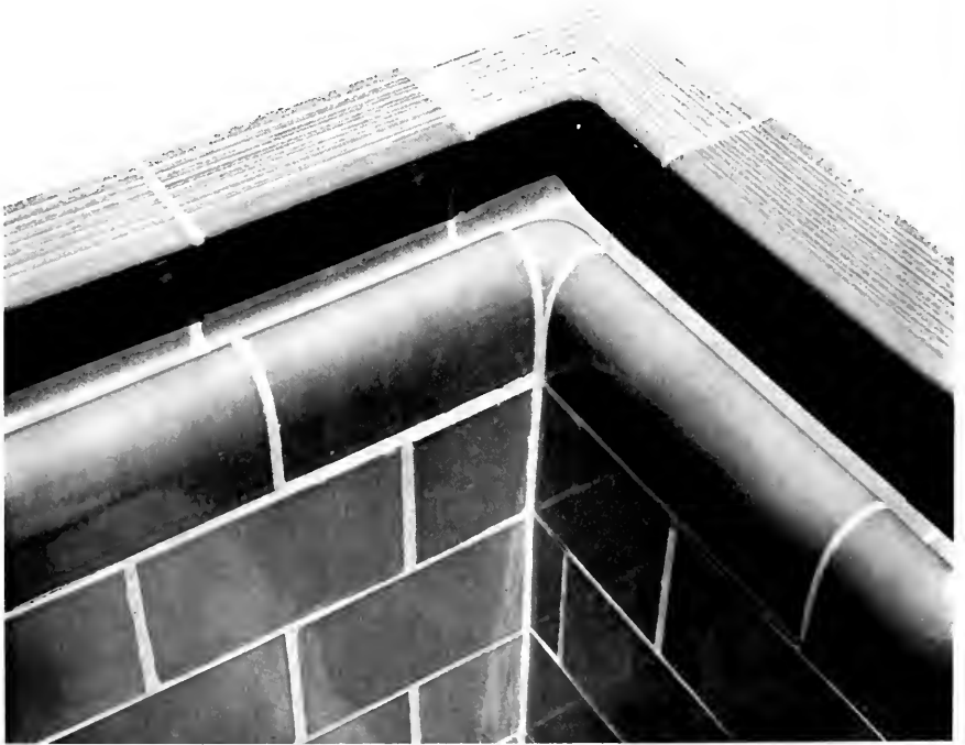
Detail of swimming pool constructed of Krafftile by Paddock Engineering Company at residence of Walter F. Foster, Hillsborough. In place of the usual mitered corners, one-piece internal angles were specified for the gutter.
