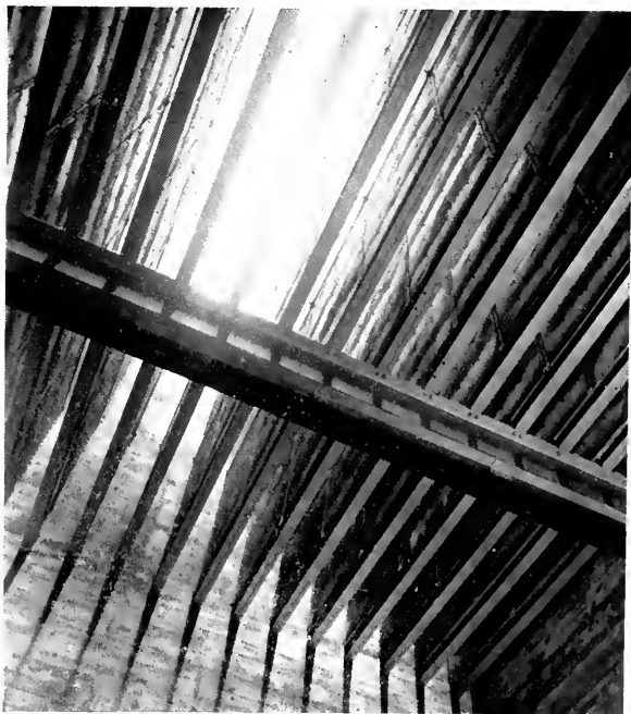
Interior view of inlet stack, looking up through the stack from a test cell floor, showing how Fiberglas bats are installed between metal sheets, and spacing of baffle plates.
