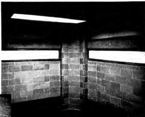
Corner of lunchroom (with glass blocks “blacked out”) shows interesting architectural details possible with Kraftile. Here, 2” thick furring tile is used on interior of the outside walls
