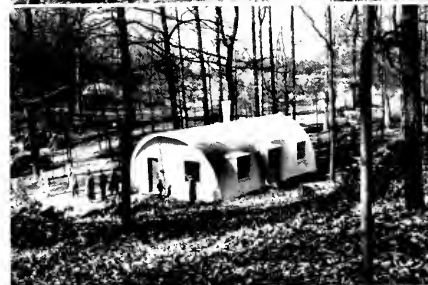
Construction methods: Pictured from top down—(1) Gunite or concrete shooting unit at left in background. Concrete base for half of housing unit in foreground; (2) Shooting Gunite onto chicken wire; (3-4) Front and side views of completed house.
