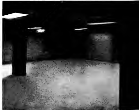
Above: Employees' Locker Room (before locker installation). Partitions for personnel rooms and offices, employees' dressing room, lunch room are 6" x 12" Kraftile "Salt-Glazed" Structural Wall Units thick with vertical cellular construction reinforced with steel grout where necessary. Partitions are glazed from floor to ceiling.
