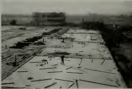
SISAL paper used to cure and protect concrete floor at United Airlines Terminal
