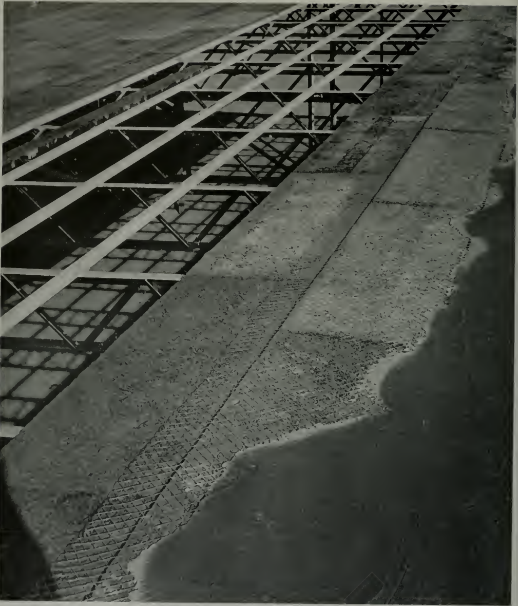
ROOF CONSTRUCTION OF INDUSTRIAL PLANT, SHOWING STEEL, THERMAX, WIRE AND CEMENT TOPPING
