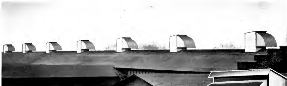
Showing blackout ventilators on roof of factory with detail of fresh air inlet louver
