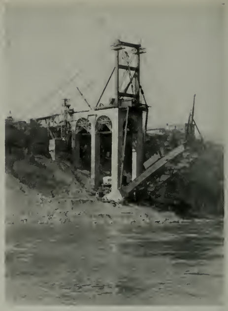
Four sections of arch rib erected with one section cantilevered beyond first tie back. Note: Rib section being moved out to derrick by means of traveler operating on near arch rib.
