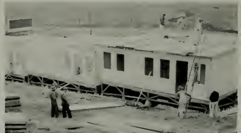
View shows prefabricated house erection in Vallejo with one roof section on the ground ready to be placed on the building.
