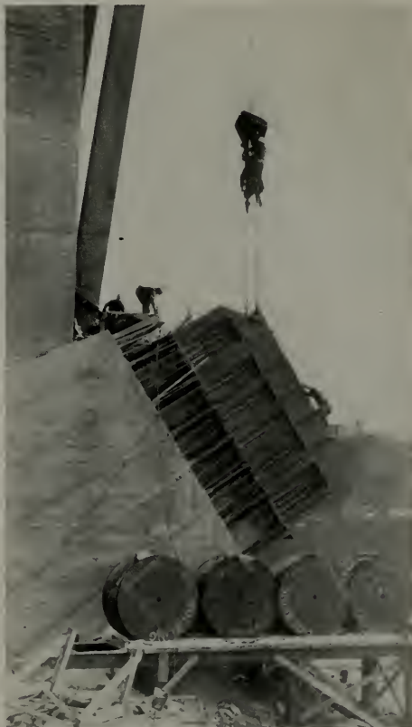
Placing of steel grillage section weighing 63\frac{1}{2} tons on anchor bolts at abutments.
