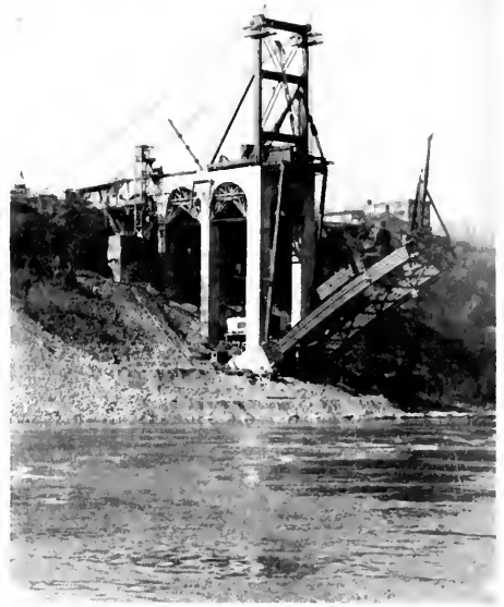
Four sections of arch rib erected with one section cantilevered beyond first tie back. Note: Rib section being moved out to derrick by means of traveler operating on near arch rib.
