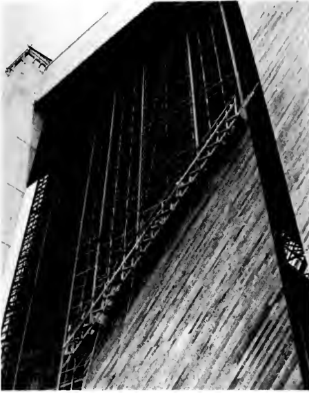
Flame-proofed wood sheathing is nailed to purlins on a steel door leaf.
