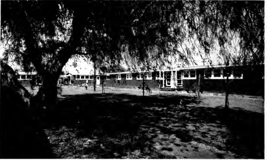
WILMINGTON HALL STRUCTURES WERE BUILT ON A JIG Prefabricated sections up to 70 feet in length were hoisted into place and nailed together.
