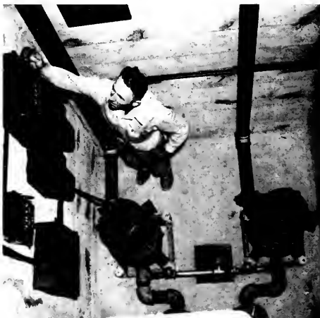
Sump Pit showing pump equipment
