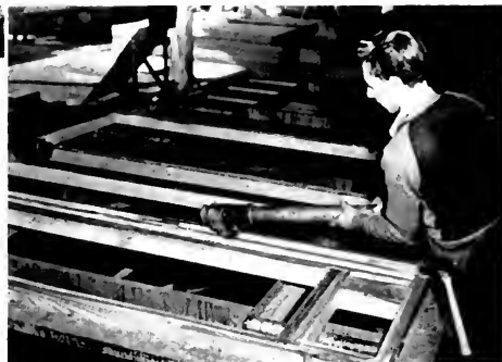
Modern methods of home construction are the result of planning by architects to facilitate erection and to make a better-built and more livable home for post-war living. Here the wall sections in a flat-bed jig are receiving glue applied by workman from a glue gun. Construction with glue not only makes stronger walls, but saves tons of nails which would ordinarily be used.
