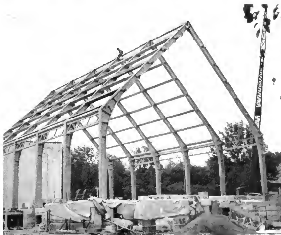
WELDED free standing framework of Church structure showing unusually high pitch of roof design.
