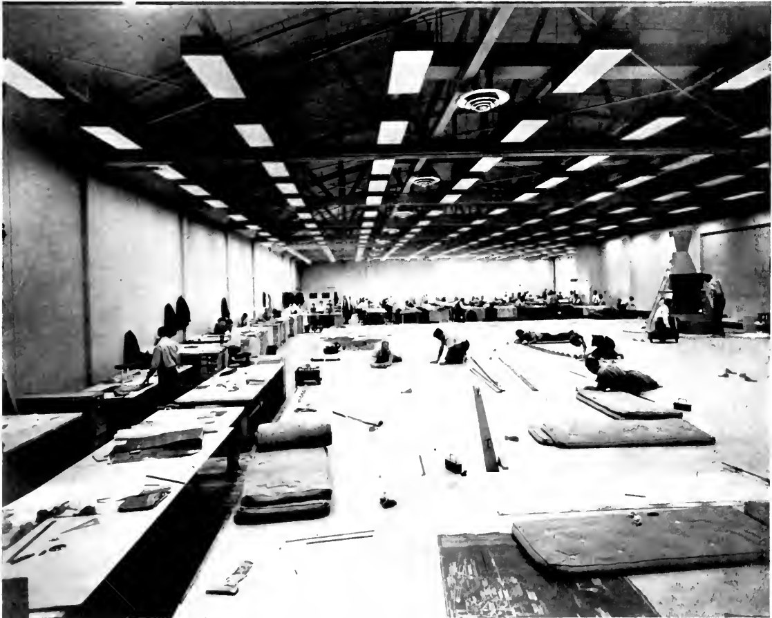
Air is distributed uniformly and without drafts over the vast floor area of this loft of the Vega Aircraft plant, at Burbank, California. By scientific air-diffusion, Anemostats (on the under-side of the trusses) insure equalization of both temperature and humidity.
