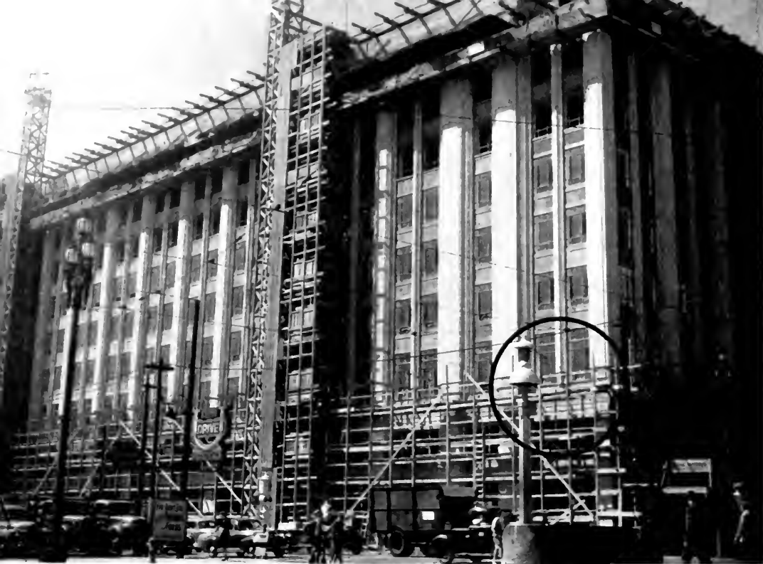
CERAMIC VENEER (TERRA COTTA) ADHESION TYPE: All plain areas are one-inch thick Ceramic Veneer applied by adhesion of the three-quarter-inch mortar coat. Anchors are used in the heavy ornamented courses only.
