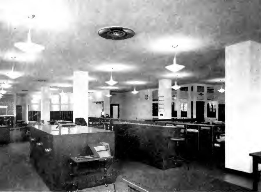
Air-diffusers insure uniform distribution of air throughout virtually all types of public buildings. Here in the Stanislaus County (California) Court House, these devices are seen on the ceiling.
