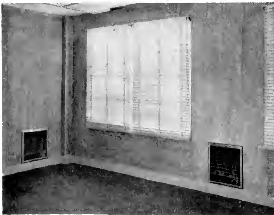
ABOVE ILLUSTRATION—Shows details of heating unit installations, in relation to floor and windows. Entire system is automatic controlled.
