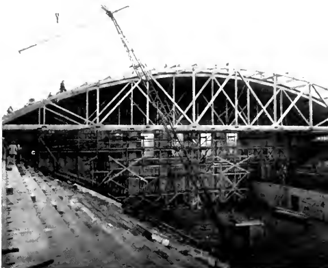
CRANE with jig boom lifts purlins into place and also lifts decking for huge roof area.
