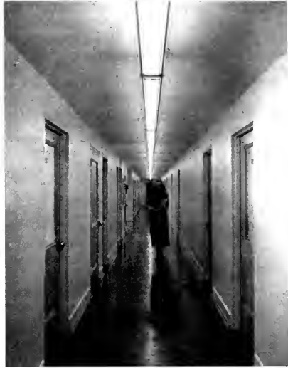
ABOVE VIEW shows corridor lighting with ceiling mounted louvered unit. Glass side panels give even distribution of light on ceiling and side walls.
