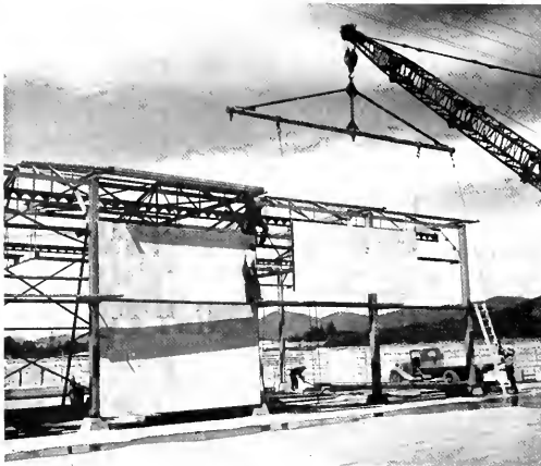
Panel of tongue and groove siding being lifted into place by crane. Section span is 16 ft. 3 in. and is 6 ft. 8 in. high.
