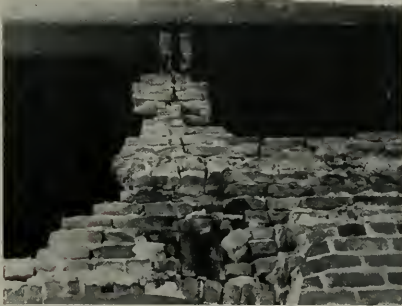
FIG. 1 Seventy year old masonry of the poorest kind in Tehachapi, California.
