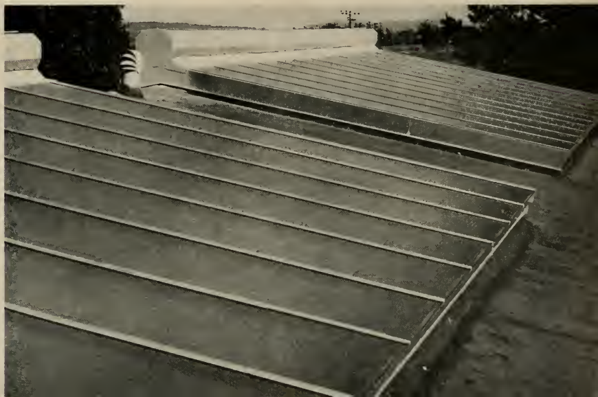
TOP VIEW of typical skylight showing aluminum glazing bars, heat resistant glass and continuous ridge ventilator.
