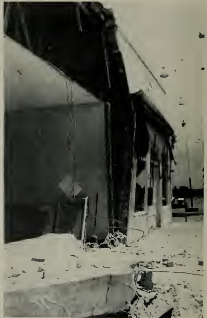
FIG. 2 Walls of this concrete block building in Arvin were not properly anchored to each other.
