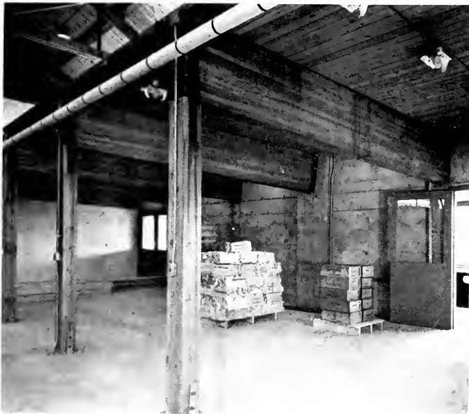
Glu-lam beams extend through into warehouse section to form timbers for support of balcony storage. Beam ends are anchored into concrete slab floor to care for extra stress in event of unusual snow load.
