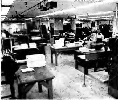
Production Department: Showing some details of building installations—wooden block floor, ventilation ducts in ceiling, and recessed fixtures for all lights.
