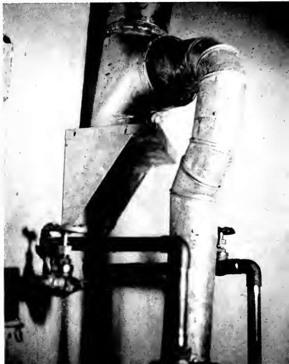
Fig. 1: Typical water heater vent.
