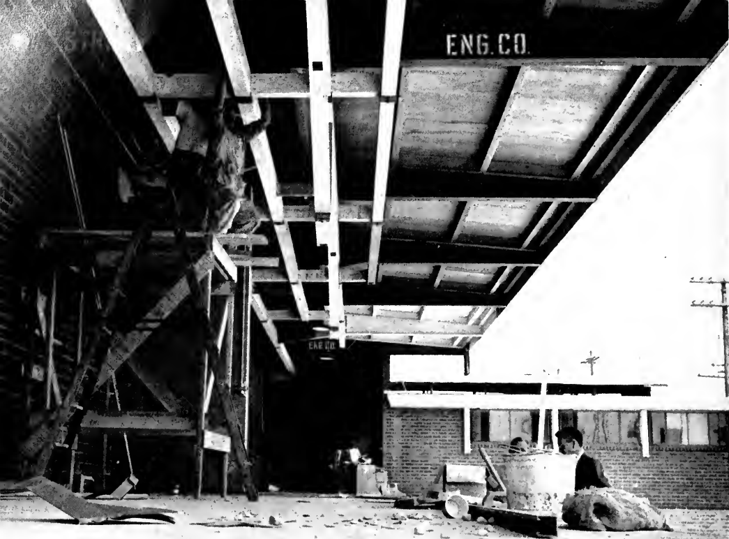
UPPER FOREGROUND shows a section of the 20 x 102 foot overhang. Four by eight foot panels of 3/4-inch tongue and grooved fir plywood used effectively to eliminate cost of expensive blocking at unsupported panel edges.
