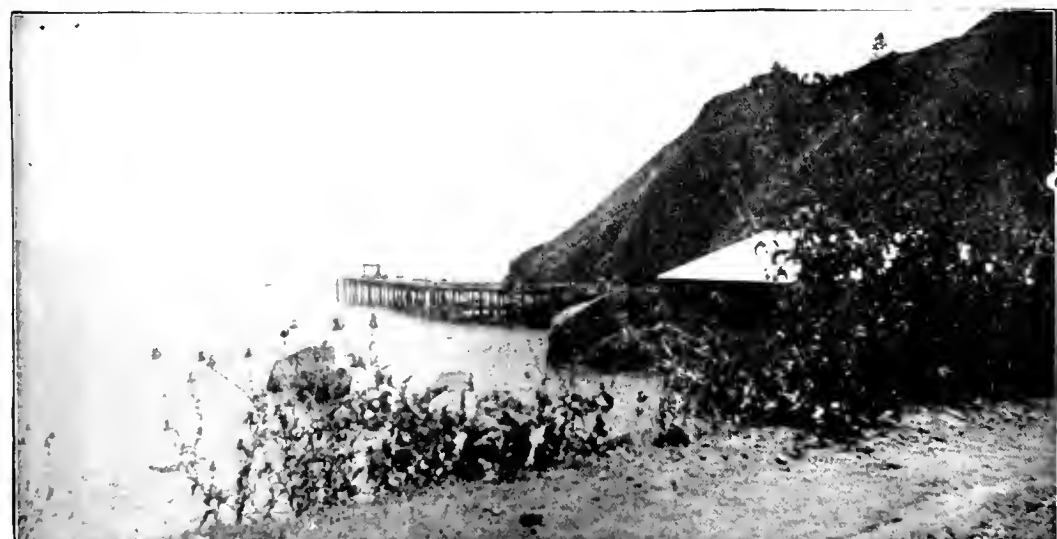
Fig. 4—Wharf recently erected at Port Orford. The piles are protected from marine borers by corrugated iron pipes.
