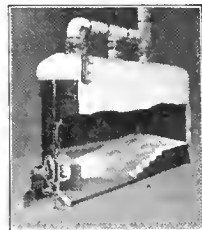
BURNER IN OPERATION
