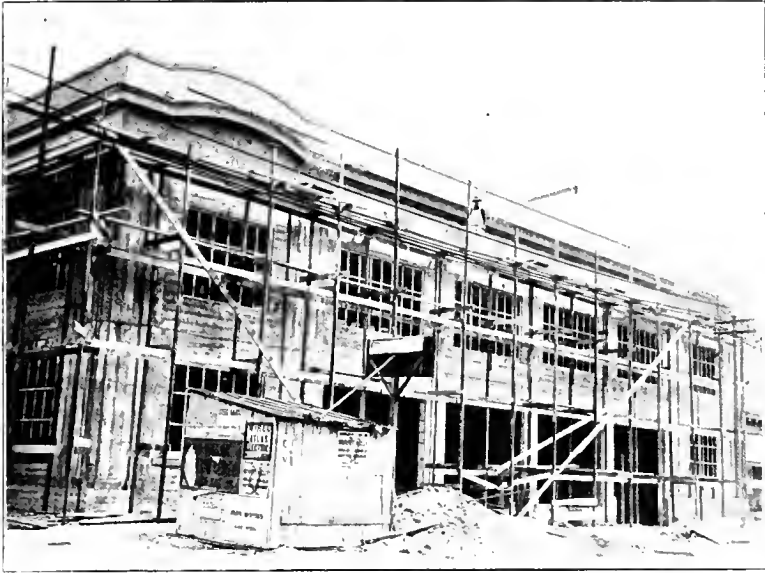
FLIMSILY CONSTRUCTED SCAFFOLD WITHOUT RAILINGS OR TOEBOARDS.
