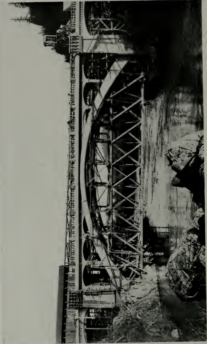
ROGUE RIVER BRIDGE, OREGON STATE HIGHWAY, SHOWING METHOD OF CONSTRUCTION. HERBERT NUNN, HIGHWAY ENGINEER; C. B. McCULLOUGH, BRIDGE ENGINEER
