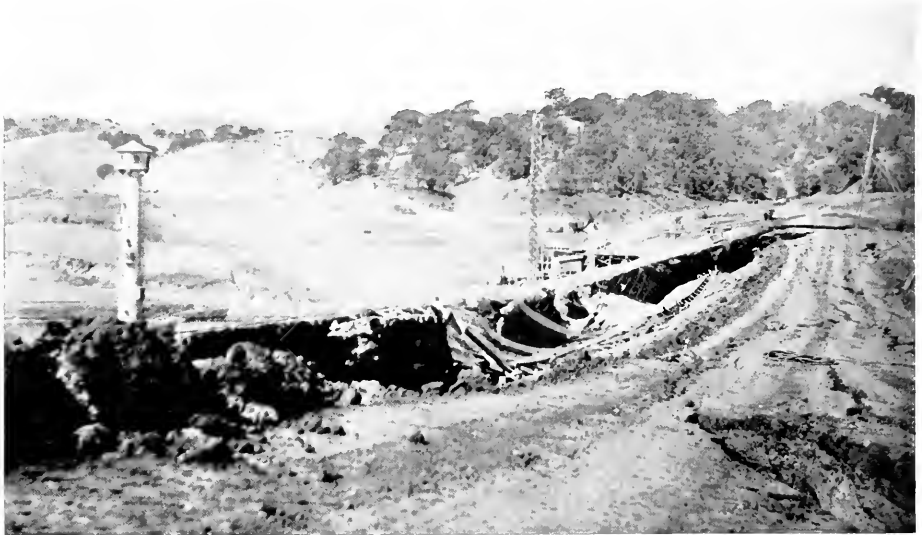
UP-STREAM CREST OF LAFAYETTE DAM, SHOWING SLIPPING OF BODY FROM CONCRETE SKIN
