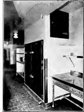
One of the Service Refrigerators
