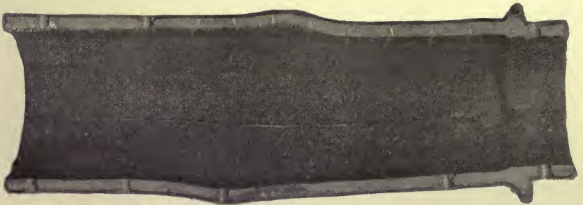
Sections of column from Western Union Telegraph Co.'s Building (Broadway, New York), showing action of fire. Removed by Jackson Architectural Iron Works.
