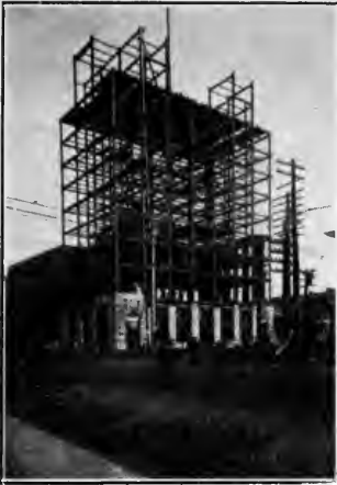
Feb. 4.—Limestone one story high and ten tiers of beams in place. Fireproofing in fourth tier.
