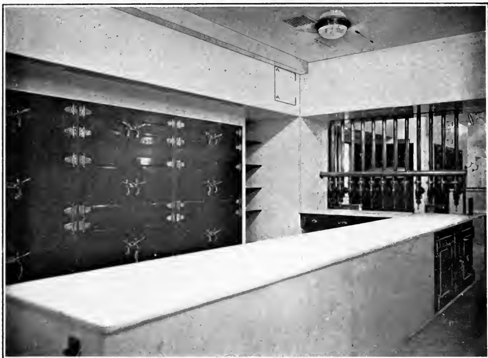
SERVICE REFRIGERATORS, HOTEL ST. REGIS. Installed by Jewett Refrigerator Co.
