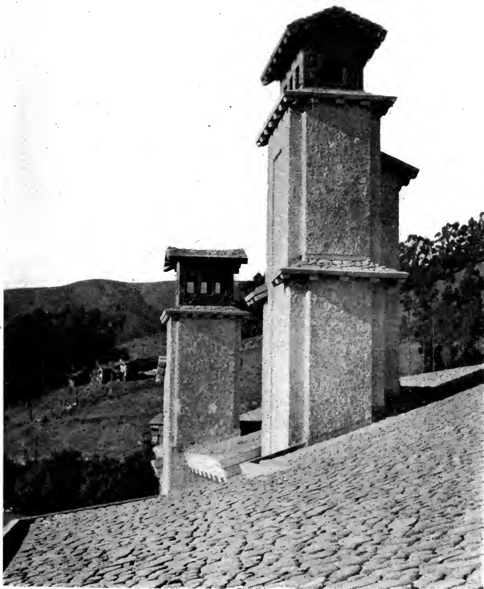
CHIMNEY DETAIL—RESIDENCE OF HENRY W. TAYLOR, ESQ., CLAREMONT PARK, BERKELEY, CAL. LOUIS C. MULLGARDT, ARCHITECT.
