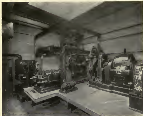
ELEVATOR MACHINERY TOP OF SHAFT.
