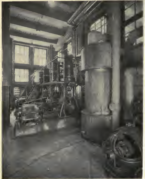
Pump Room—Ice Machine. THE CURTIS BUILDING.
