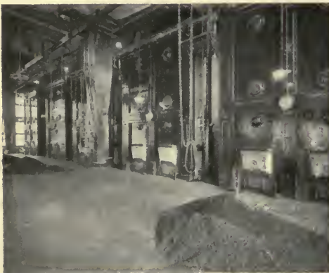
THE BOILER ROOM.
