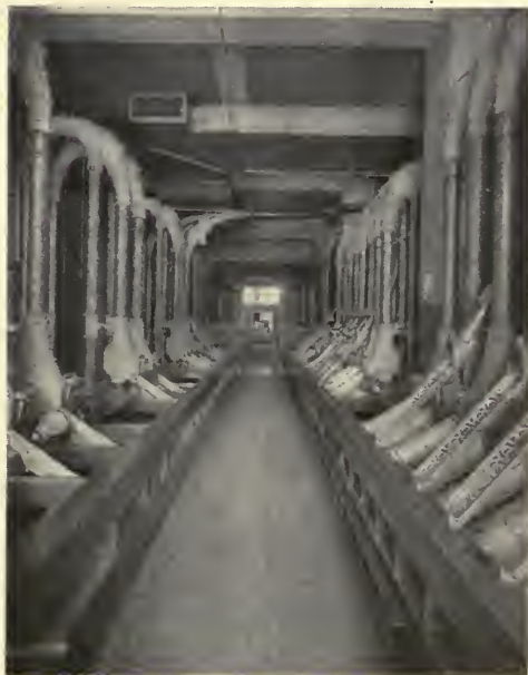
STORE SERVICE TUBE ROOM.
