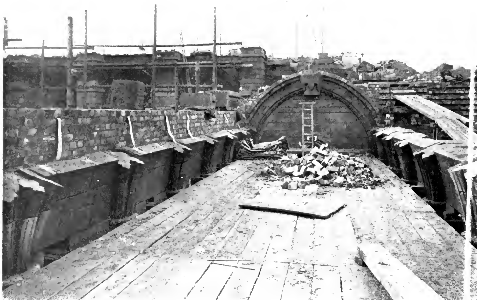
AMBULATORY AT BACK OF ALTAR—THE CATHEDRAL CHURCH OF LIVERPOOL. G. Gilbert Scott, Architect.
