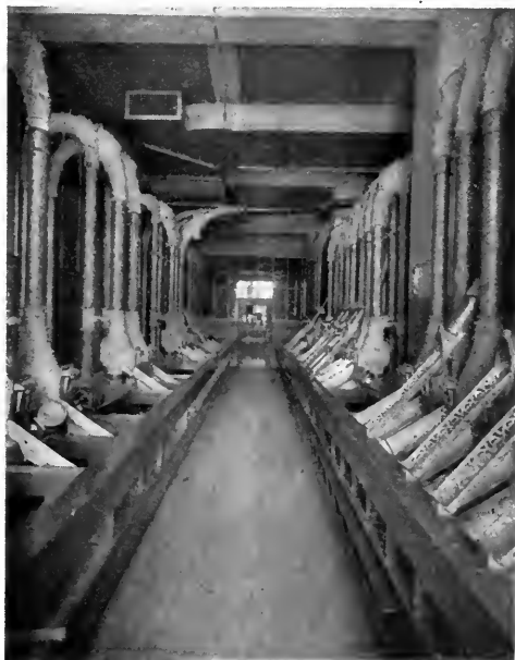
STORE SERVICE TUBE ROOM.
