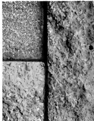
Corner Blocks Are Finished in the Same Way That Stones Are Quarry Faced. The Others Are Finished With the Pointer.
