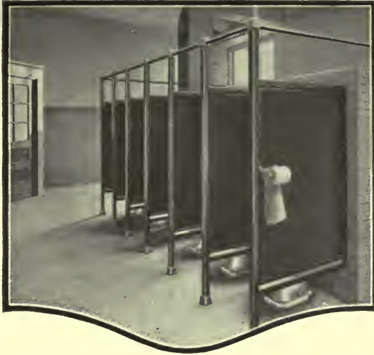
Sanymetal in the Harding Grade School, Youngstown, O. Kling, Zenk & Kling, Arch.
