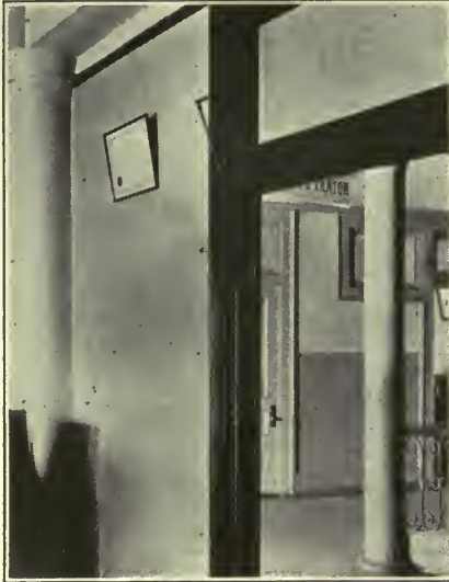
Moore Building, San Antonio. Partitions are made of 27-gauge Kno-Burn with channels 12" on centers.
