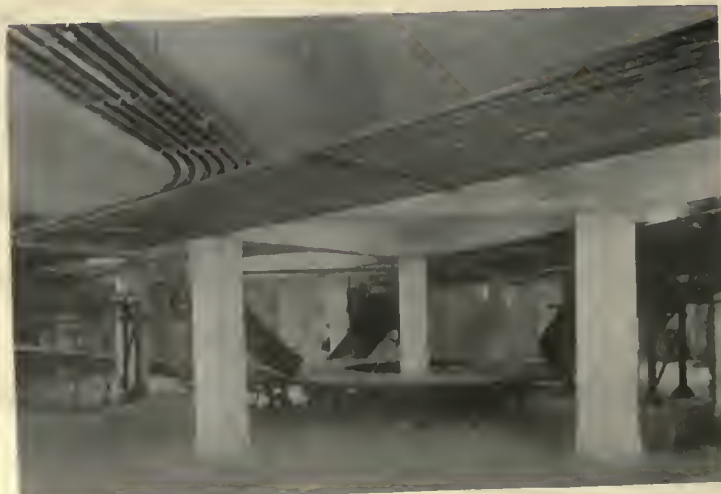
Parcel Conveyers and Rotating Table in Basement. Cash-system tubes are to be seen hung from the ceiling above.
