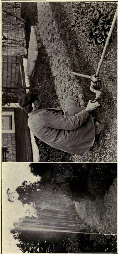
PLATE 14.—(Left) Modern irrigation can be used almost anywhere about the grounds to keep them green and flourishing throughout the summer. When the water is turned off, a line arranged like that in this picture is almost invisible. (Right) This shows the valve by which the water is turned on and off and the special fitting with the strainer and handle by which the line is revolved from one side to the other, adjusting the spray to any position desired over a plot forty to fifty feet wide and as long as the line of pipe. Where wanted, an automatic turning device takes the place of the turning handle.
