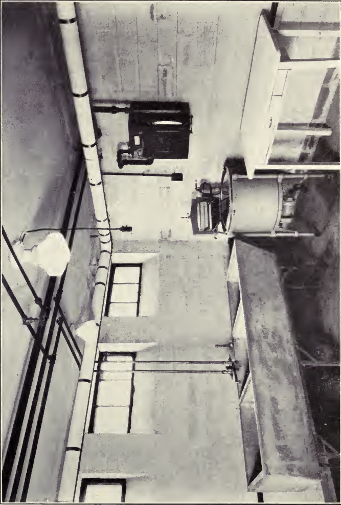
Fig. 43.—The laundry tubs have their individual light directly above and the second unit with its service outlet takes care of the ironing needs.
