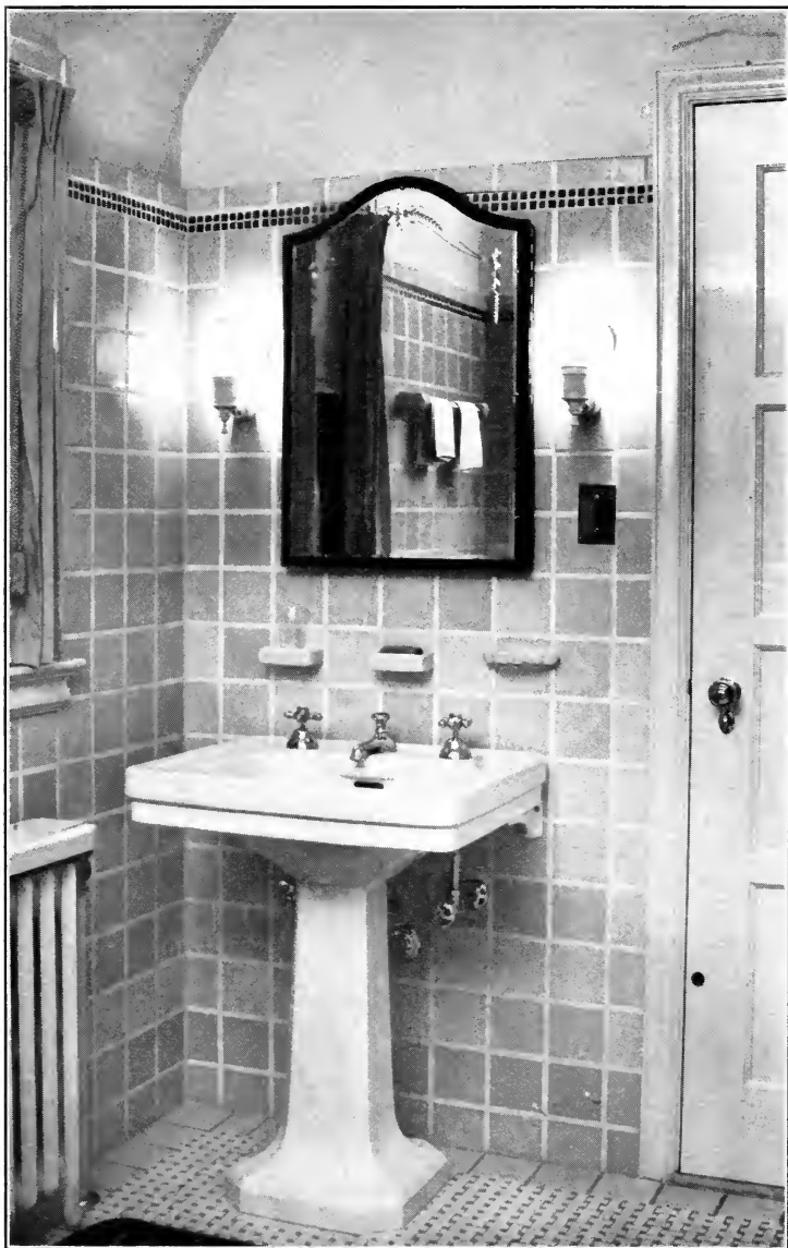
FIG. 42.—Carefully shaded wall brackets at face height on both sides of the bathroom mirror constitute very satisfactory lighting.
